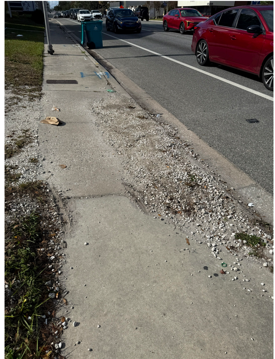
Figure 69: Debris and Sediment on Sidewalk; Garbage Receptacle in Bike Lane
