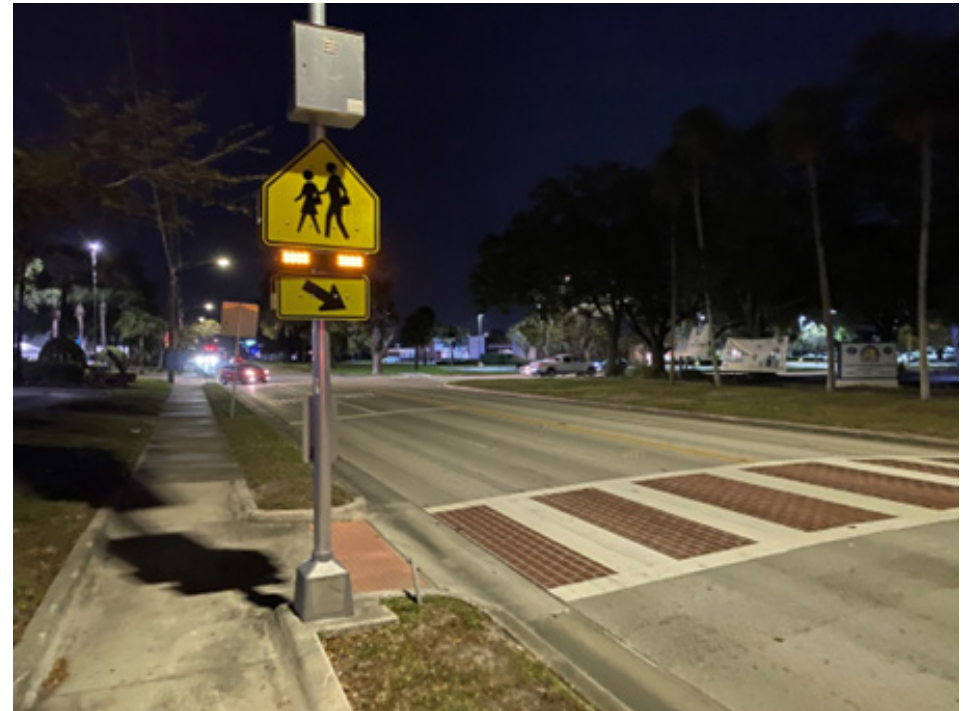
Figure 103: Rectangular Rapid Flashing Beacon Assembly on Primrose Drive
