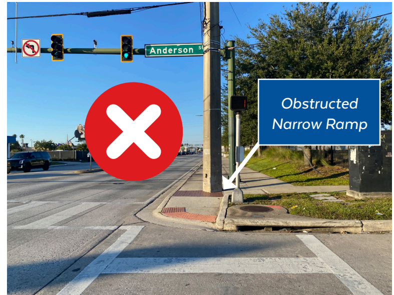
Figure 60: Obstructed and Unobstructed Curb Ramps on Orange Blossom Trail
