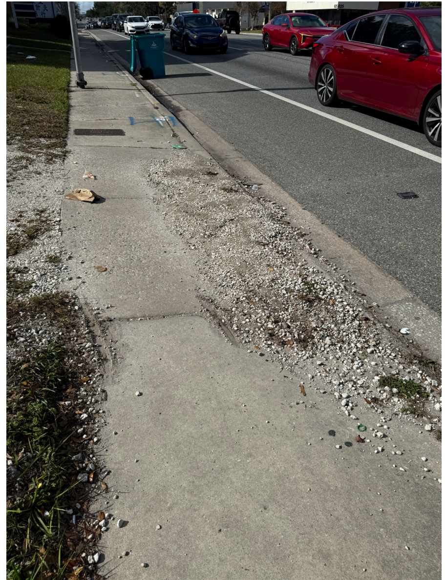
Figure 63: Debris and Sediment on Sidewalk; Garbage Receptacle in Bike Lane
