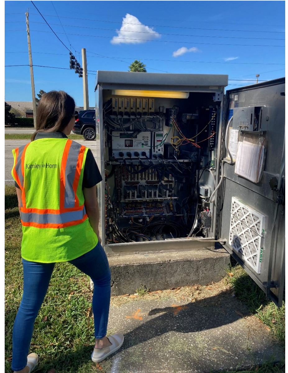
Figure 67: Signal Timing Modifications inside Controller Cabinet
