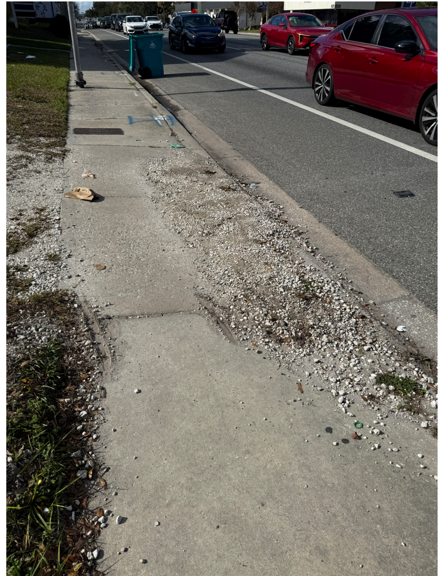
Figure 76: Debris and Sediment on Sidewalk; Garbage Receptacle in Bike Lane
