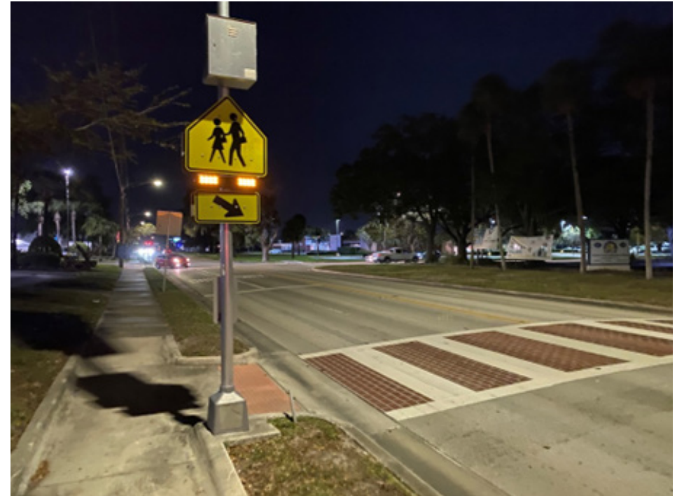
Figure 91: Rectangular Rapid Flashing Beacon Assembly on Primrose Drive
