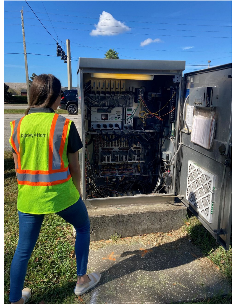
Figure 66: Signal Timing Modifications inside Controller Cabinet
