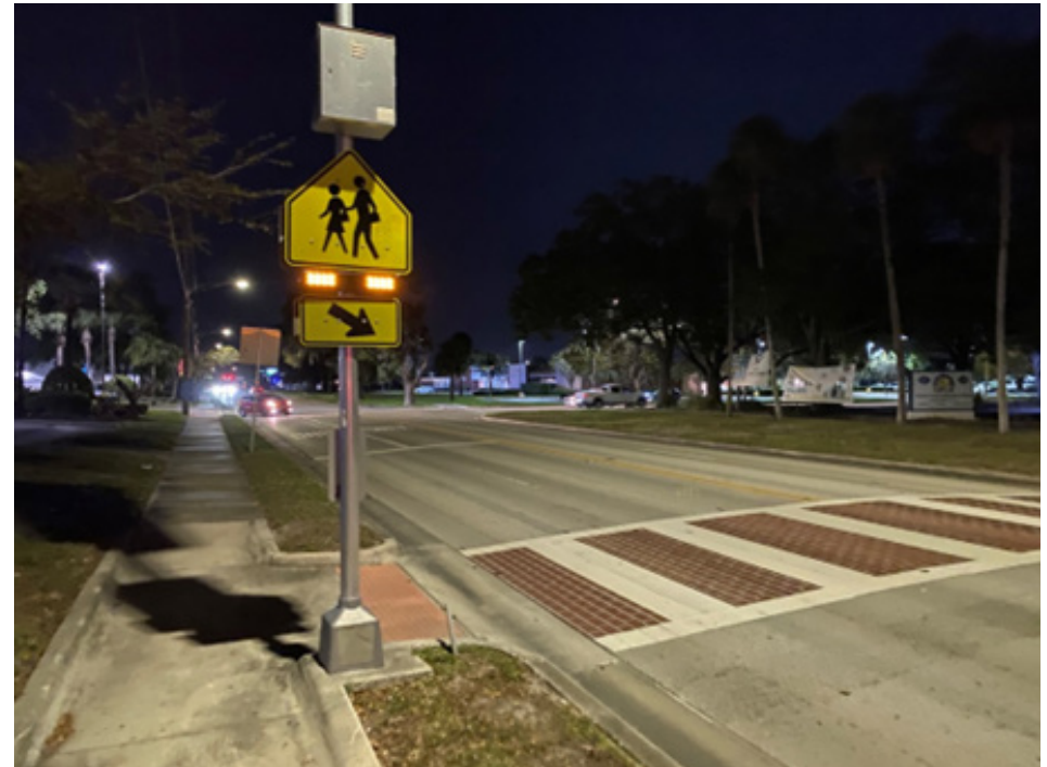
Figure 89: Rectangular Rapid Flashing Beacon Assembly on Primrose Drive
