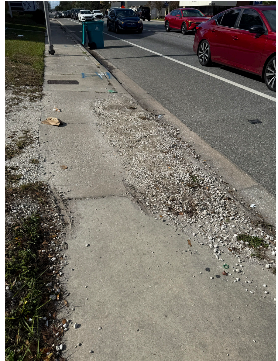
Figure 60: Debris and Sediment on Sidewalk; Garbage Receptacle in Bike Lane
