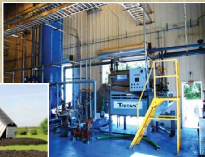
Wastewater operations and equipment
