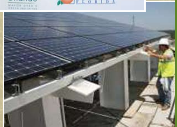
OUC's new roof-mounted 32-kilowatt photovoltaic system
