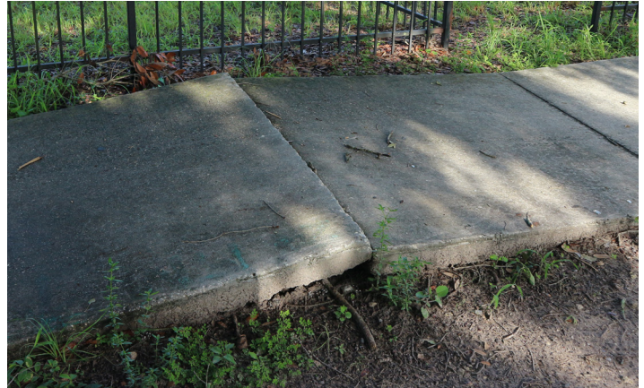
Figure 19: Sidewalk in need of maintenance.
