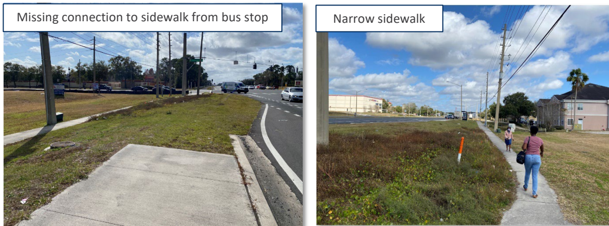
Figure 12 | Raleigh Street at Kirkman Road Observations and Concerns
