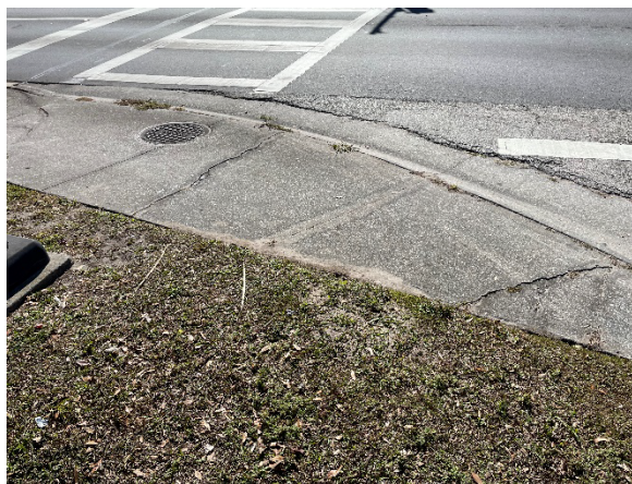
Unclear, unseparated curb ramps.
